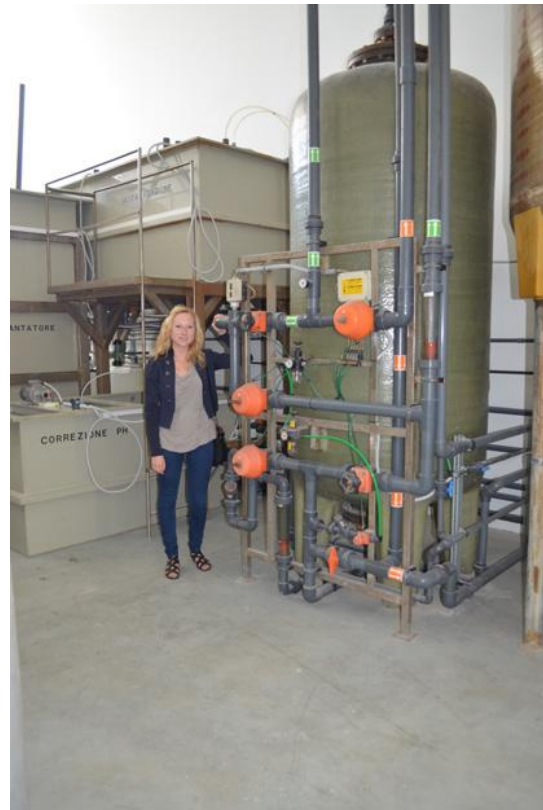
Fig.12: Part of an advanced system for wastewater treatment (after the process of electroplating)
