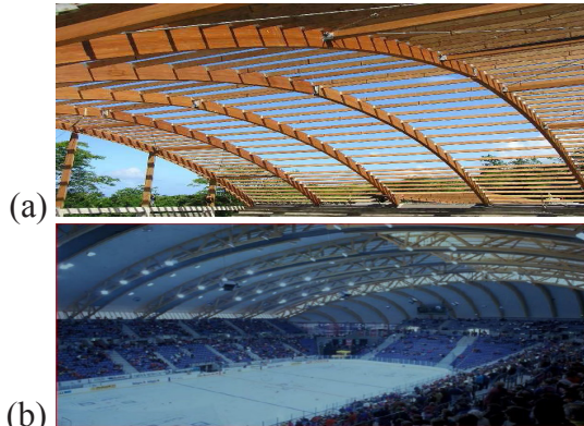
Fig. 1. Arch-type timber structures: (a) of sport stadium Majuro; (b) of Hakona hall [8].
