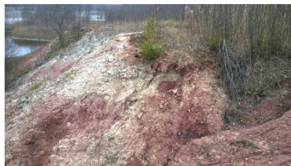
Fig. 3. Dolomite landslips in the Kuprava quarry wall.
