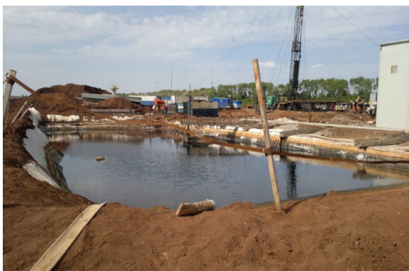
Fig. 1. The two-section mud pit.
